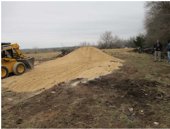
Blending excavated material with agricultural lime stabilized the contamination and reduced disposal costs.
